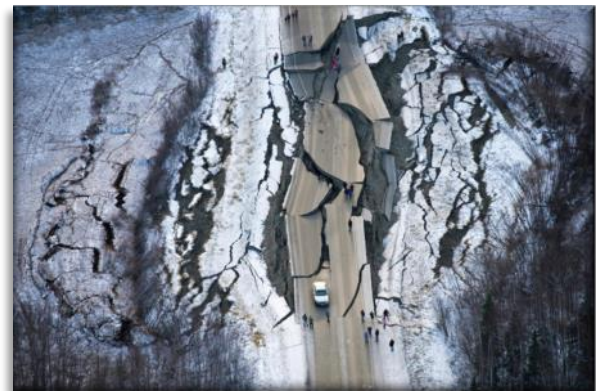
Aerial photo showing damage on Vine Road south of Wasilla, Alaska after the November 30 201 earthquake.
